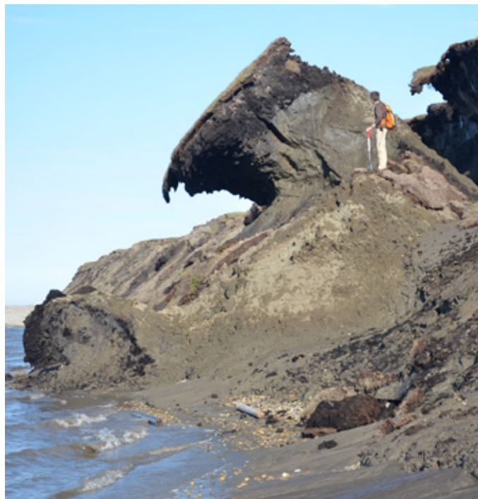
Eroding coastline near Barter Island on Alaska’s North Slope. (B. Jones, USGS)
