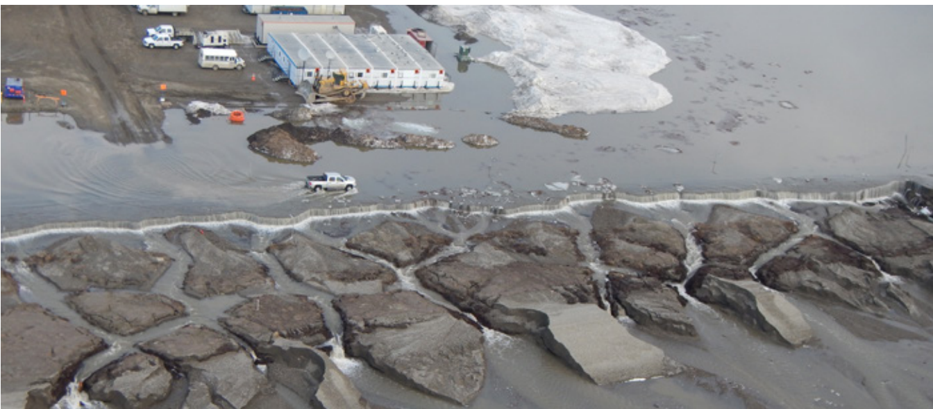
Spring flooding from the Sagavanirktok River overruns the Dalton Highway at Mile 413. (J.Organek, ADOT.)
